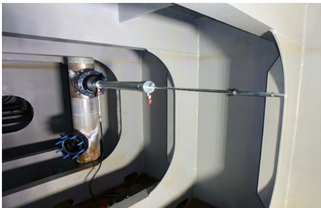
Figure 2. Methods used to isolate and repair sea valves by ROV and by internal isolation.
