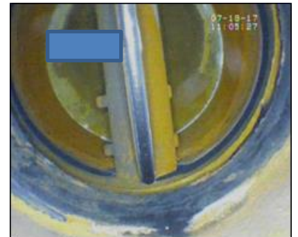
Valve Inspection with ODIN Camera
