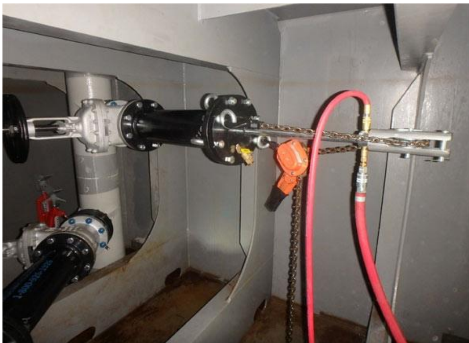
Figure 2. Valve and pipe isolation.
