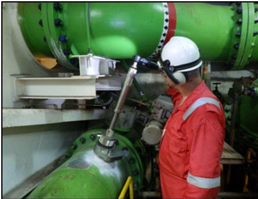
Figure 1. In service isolation valve inspection.
