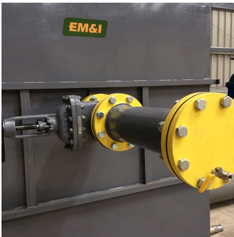
Figure 4. ODIN access port to seachest and valve.
